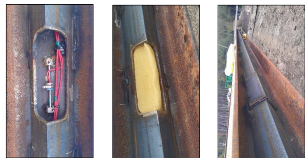
a) Covering the cables, and sensors by a fire resistance fabric b) Adding extra piece of protecting angle
