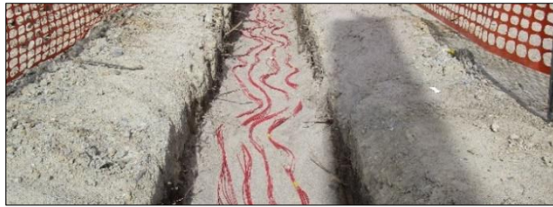
Figure 10. Serpentine layout of cable bundles
